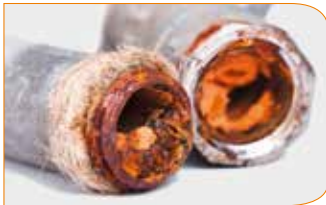
Magnetite sludge in pipes and valves
