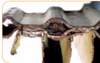
Radiators clogged by deposits
