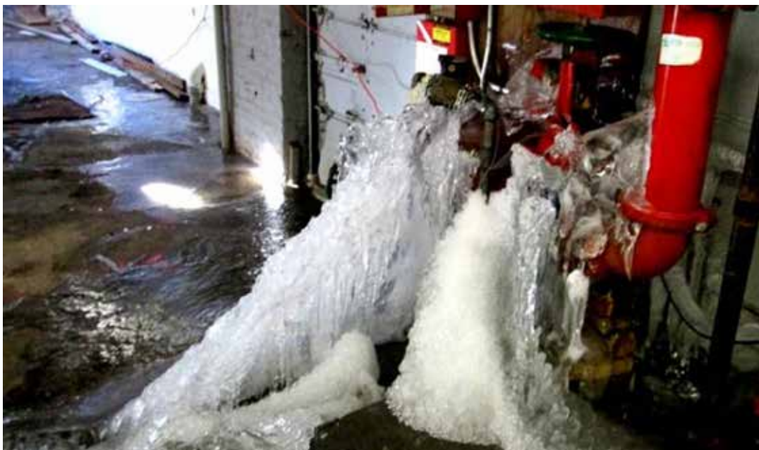
In this example, after a power supply breakage, the valve remained at its closed position not enabling a minimum flow to prevent pipe freezing. This led to repair costs 242 k€ and a shutdown of the HVAC system.
